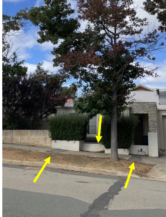
Figure 6 - Lifted and repaired footpath, cracked wall
