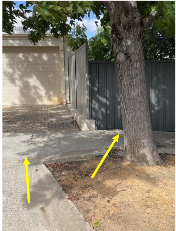
Figure 8 - Tree 7 Cracked and lifted foot path, uneven driveway
