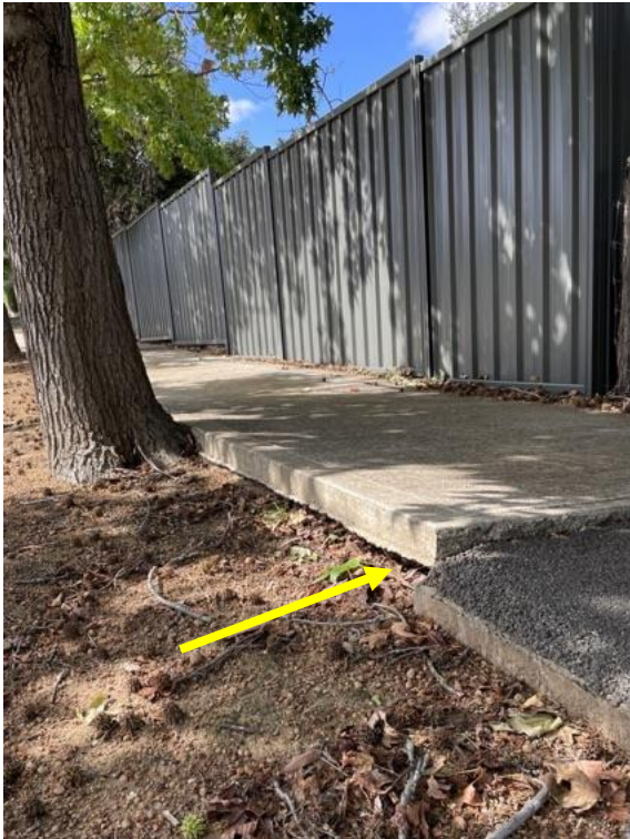
Figure 7 - Tree 9 Lifted footpath
