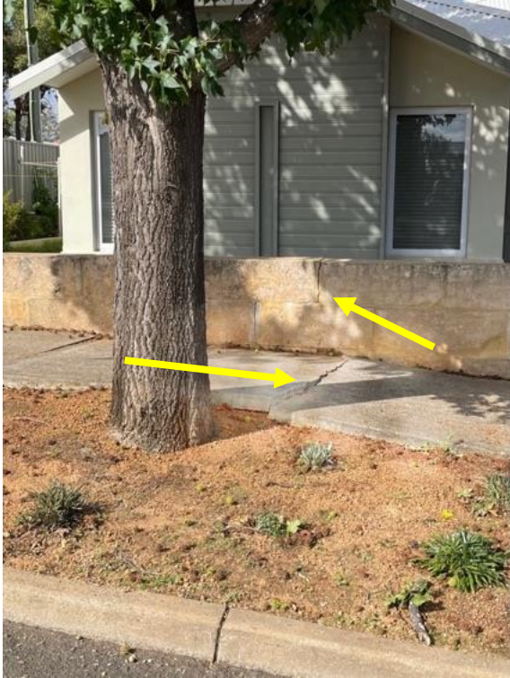
Figure 5 - Tree 2 Cracked lifted footpath, cracked wall
